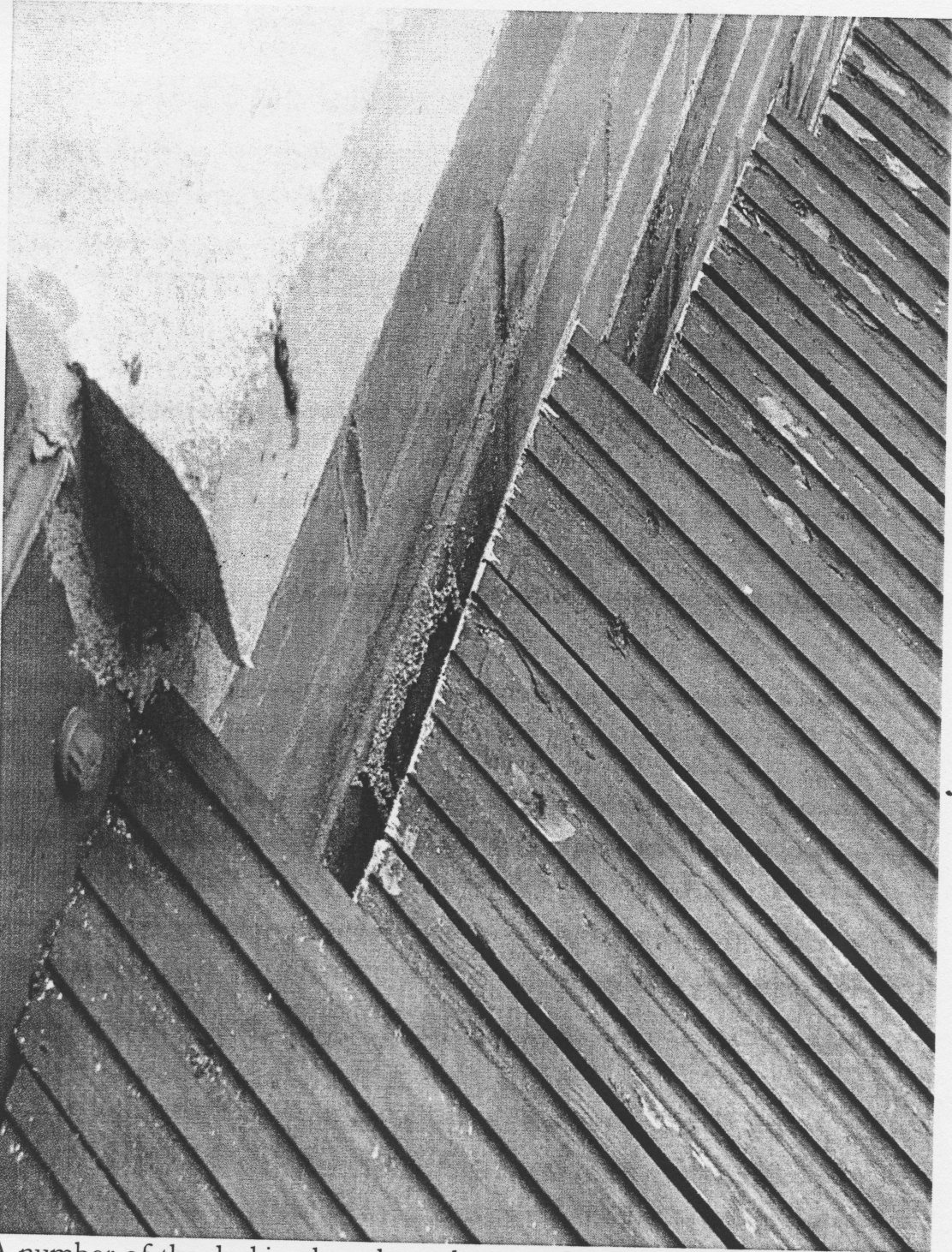
A number of the decking boards are loose and rattle underfoot. The standard of cutting out of the edges is very poor and irregular.
