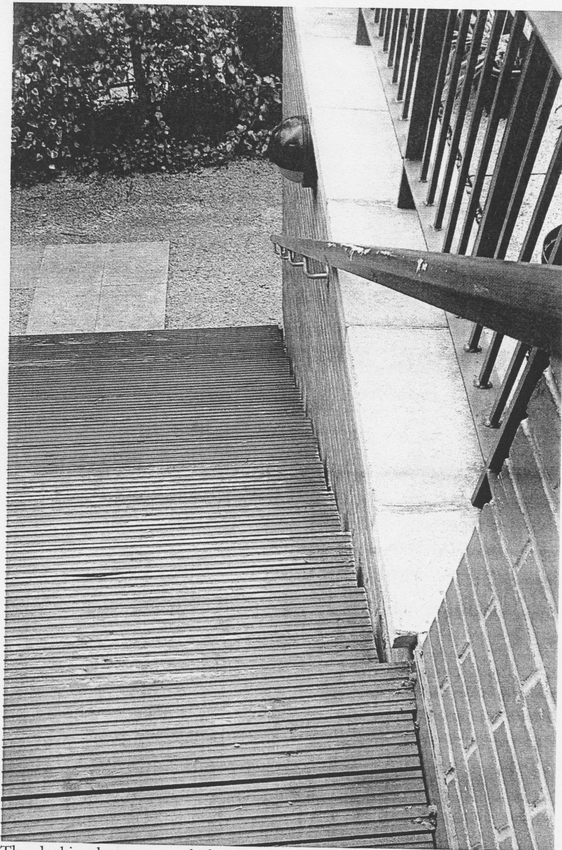
The decking has apparently been giving problems with water ingress to the edges of the steps.
