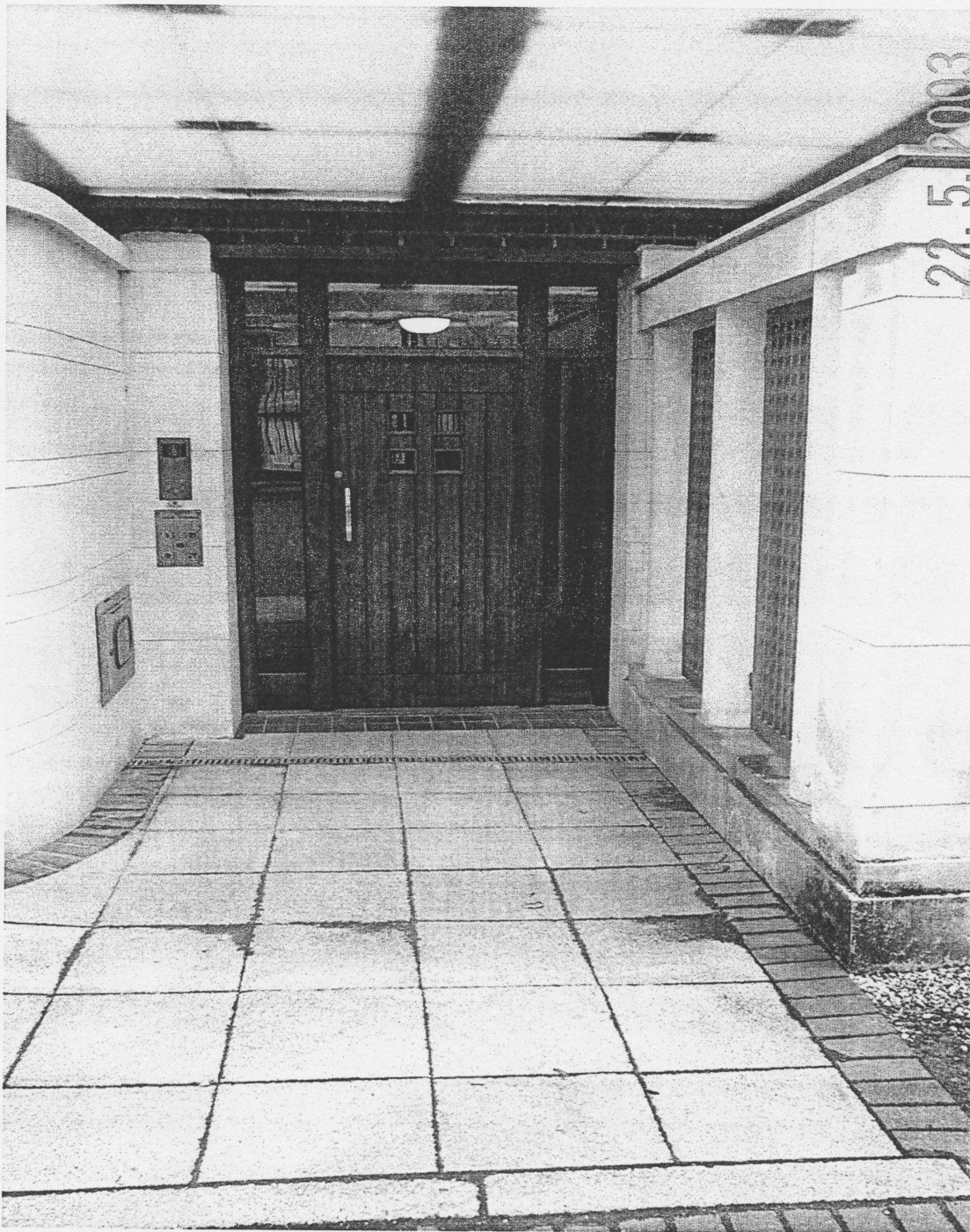
Mould growth and damp staining to stone pier.
